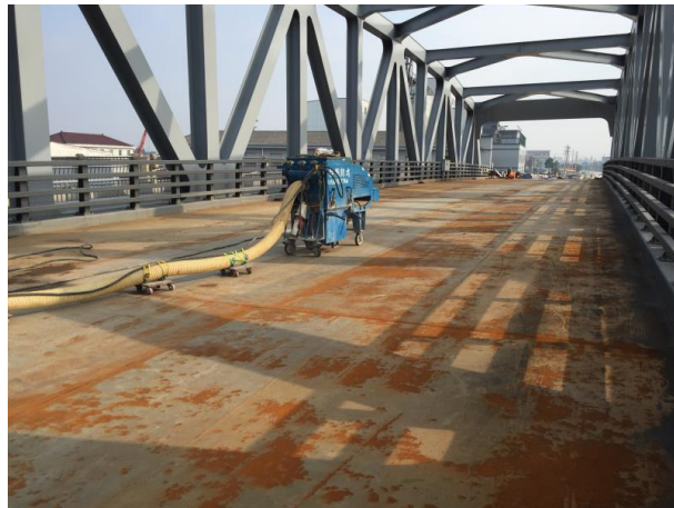
锈渣粉尘回收
